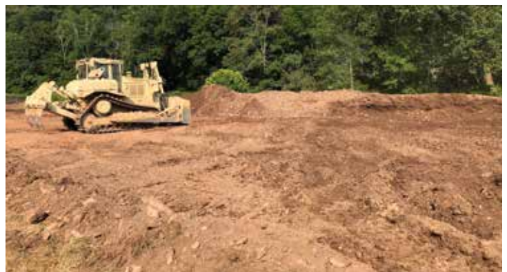
The Army Reserve Unit used removing the berm as a training exercise. Less experienced soldiers removed the bulk of the berm, but left an edge (you can see it here in front of the dozer). The more experienced operators came back through to remove the edge and get the site to its final grade.
