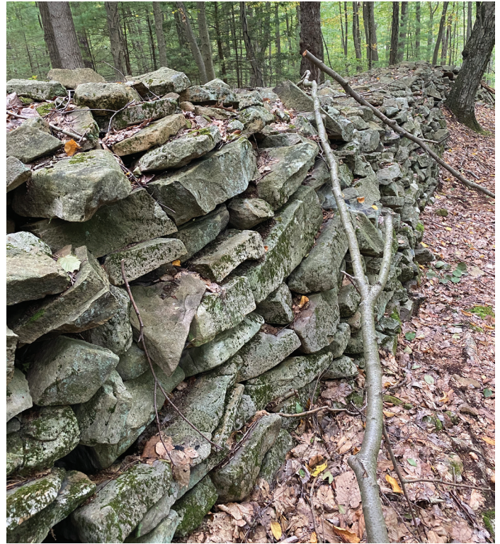
THE MORGAN VALLEY EASEMENT stone wall is the largest I have encountered on any of NPC's easements so far this year.
