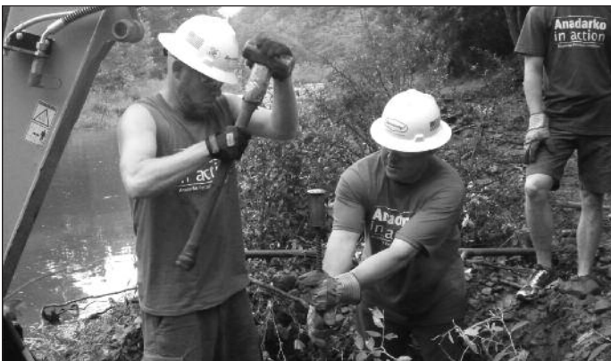
Using a sledge hammer and a driving head, two Anadarko employees start driving at 4-foot piece of rebar.
