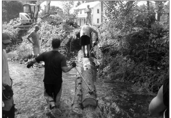
Construction provides an opportunity for education. At this site on Rapid Run (Union County) neighbors (the women on bank, and the gentleman on right) watch as Tyler Neimond drills holes for the rebar, and Keith Beamer gets ready to start rebar with sledgehammer.
