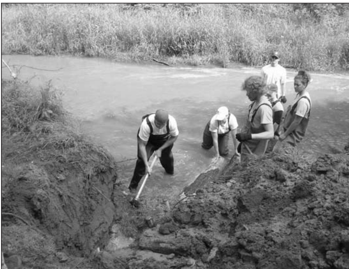
After the trench is created in the bank, and the log placed in the trench, volunteers use sledgehammers to pin the log with rebar. Here Lycoming College Cleanwater Institute interns pound the rebar in.
