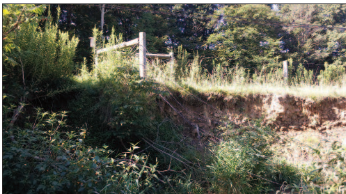
Before the project the stream was eroding toward a heavily used road.
