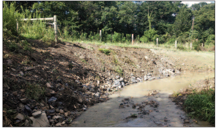
After the project, the bank has been regraded to reduce erosion and restore functionality during high water.
